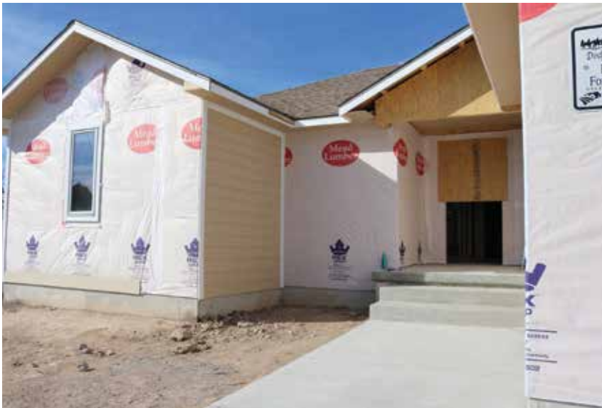
The newest home on Mulberry Circle in Dodge City is about half complete.
