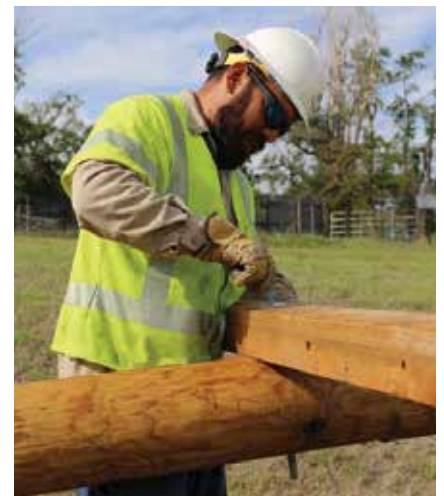
Vidal Moreno Jr. frames a crossarm, which helps support the wire. Each pole has to be framed with cross arms before it can be set.
