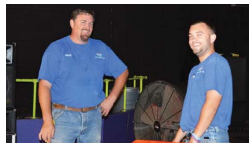
Victory Electric donated the labor to upgrade and install new lights at The Alley to benefit the afterschool program. The electricians, Harold Bogner (left) and Ross Adams replaced non-working lights, outdated fixtures and security lights.
