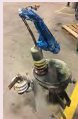
A metallic balloon landed on a transformer and caused blinks and disrupted service for members in May.
