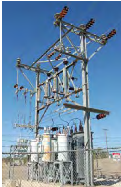
Victory Electric has 53 substations to get power to your homes and businesses.
