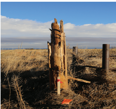
Winds from November 16 caused pole damage and some poles to break completely causing power outages.
