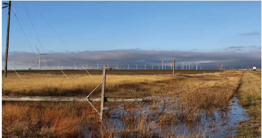
Downed power lines created outages for several members following the November 16 storm.
