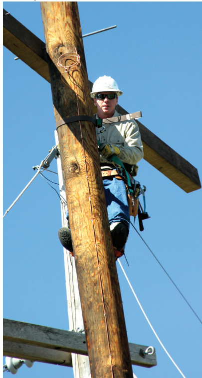
Justin Straight makes sure the arm is in the correct position before installing.
