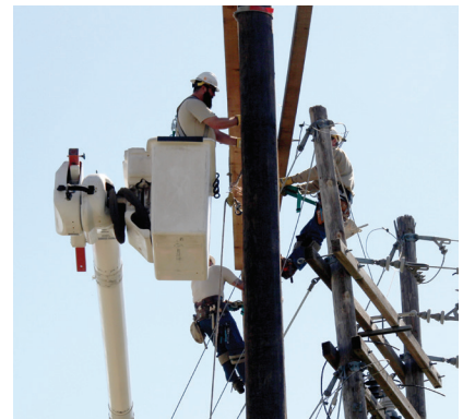
Mikey Goddard works from the bucket truck to place the cross bars in the structure.
