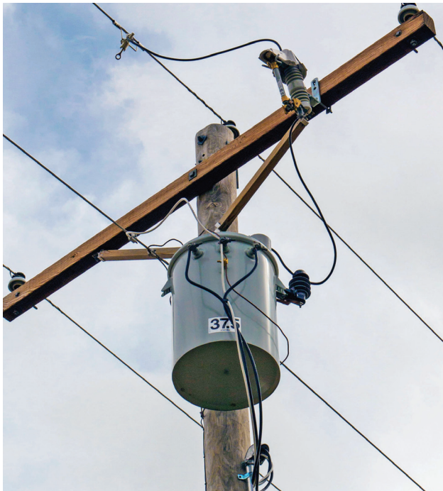
Transformers reduce voltage as it travels to your home, making it safe to use.
