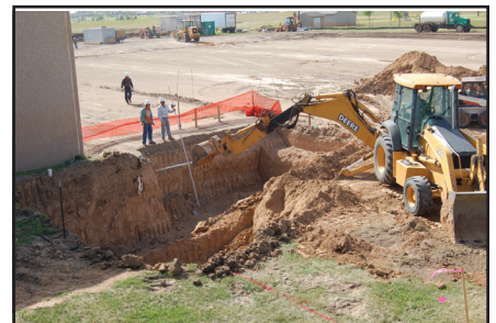
Construction crews dig a hole to make room for the new basement of the Victory Electric office building.
