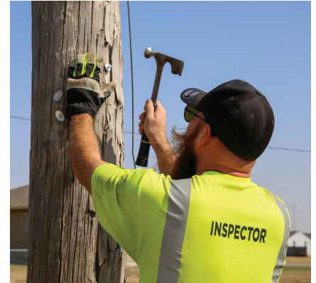
After boring, Sundance PPI inspectors use a hammer sound test to see if a decayed pocket extends above the ground line.
