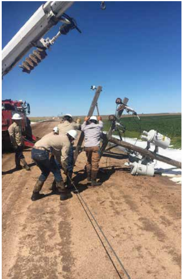
Victory Electric linemen move a broken pole out of the road.
