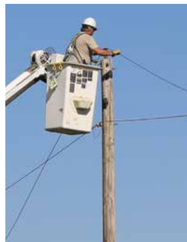
The storms caused miles of line to be knocked on the ground that had to be reattached. Lineman Dave Lowry attaches wire to the pole.
