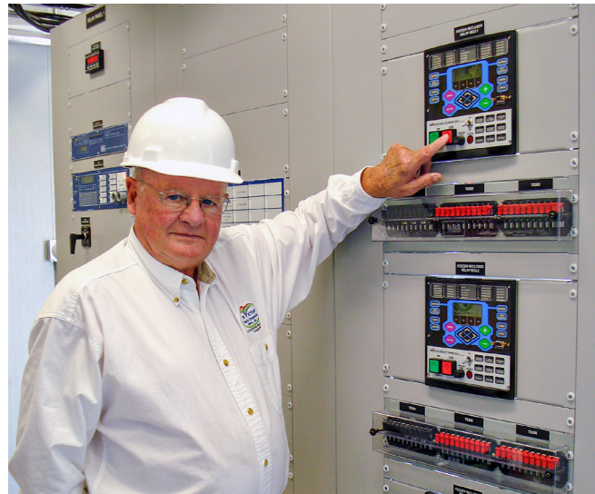
Loren Ochs flips the switch to energize the Loren Ochs Energy Center substation in 2010.
